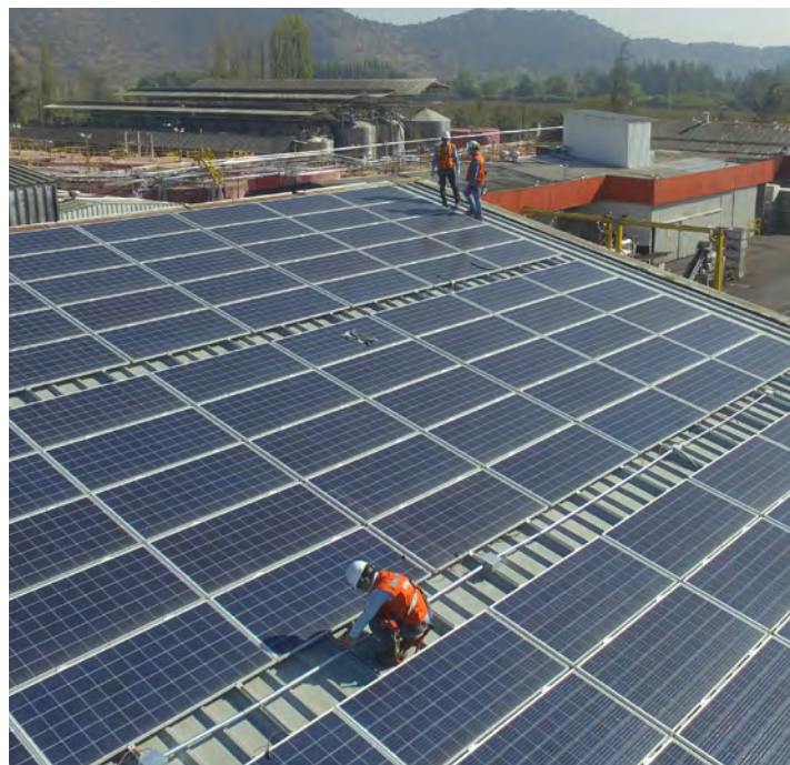
Cintac has installed over 100,000 m 2 of rooftop photovoltaic plants, such as the one in Viña Lourdes.
