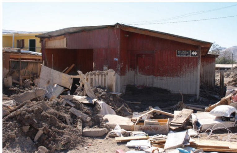
Photo 6: House obstructed by debris left by the alluvium, Copiapó, March 2015 (Photo: C. Jiménez)
