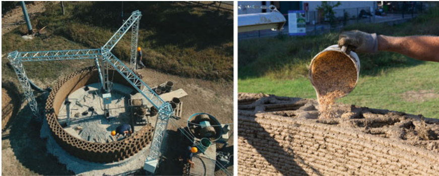
Fig. 9 Construction of the Gaia House [33]. a 3-D printing of the outer walls with ABM based mixture, b vertical cavities of the 3D-printed wall are filled with rice husk for insulation
