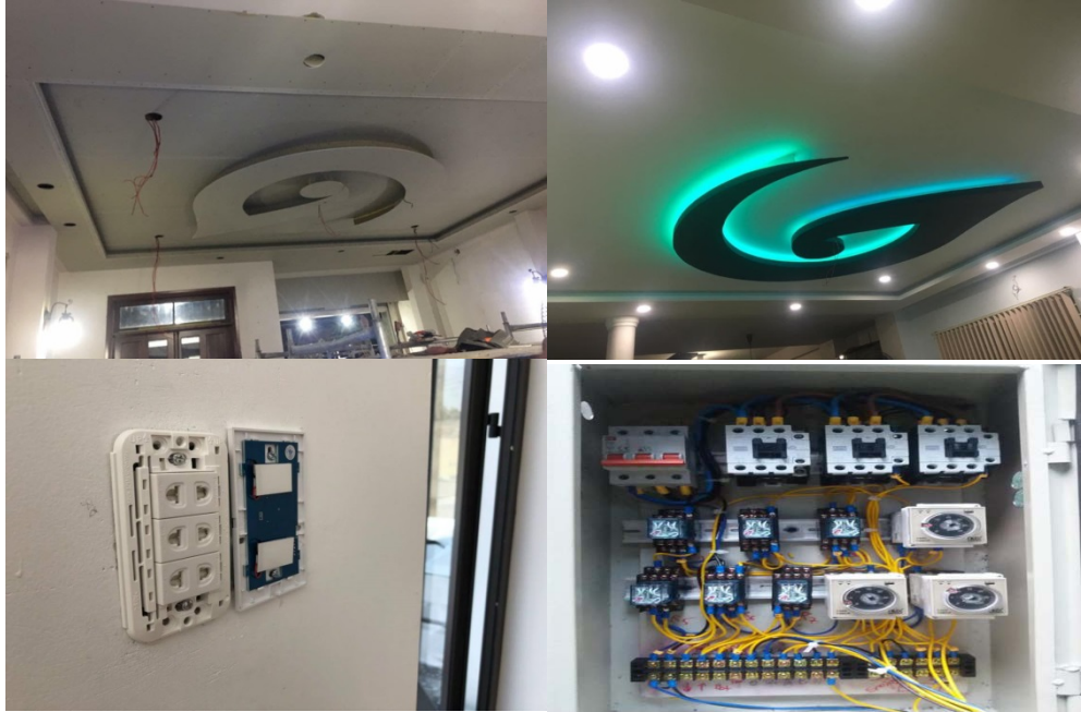
Figure 4. An example of smart home installation
